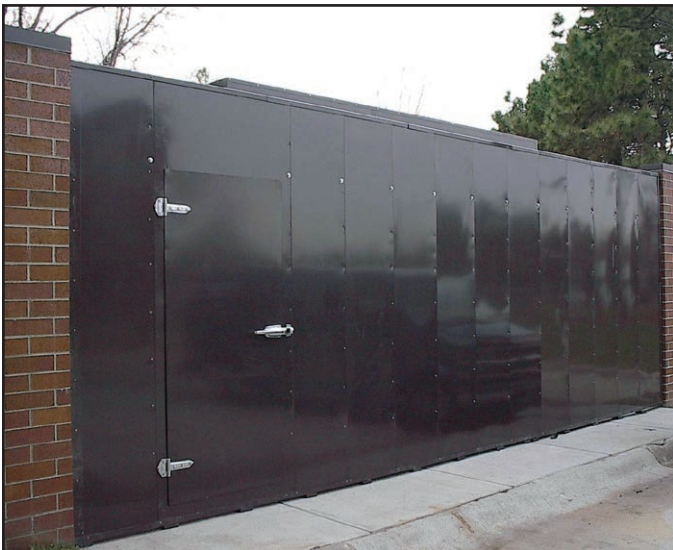
Air-cooled chiller attenuation systems
